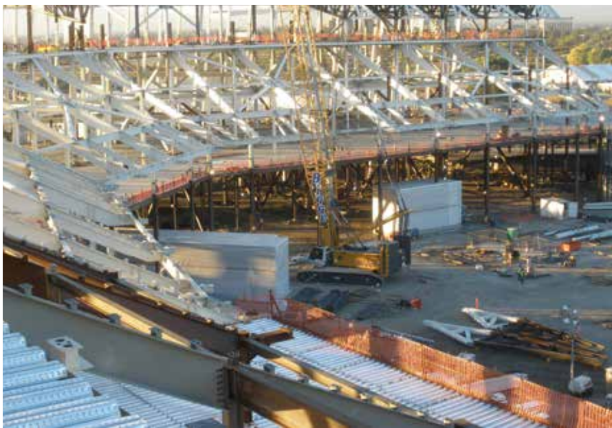
About 1,200 workers were on the construction site each day to meet the ambitious target date for completion.
