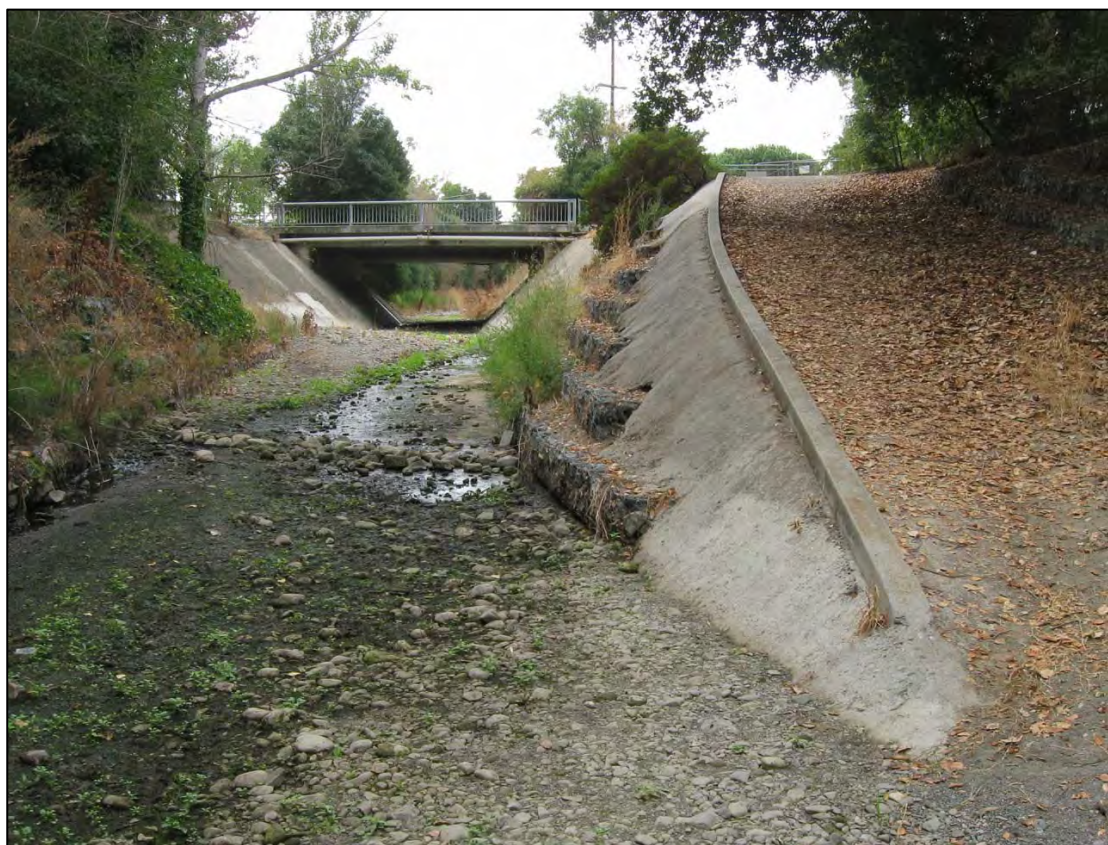
View looking upstream at the Kiely Boulevard bridge and maintenance access ramp.
