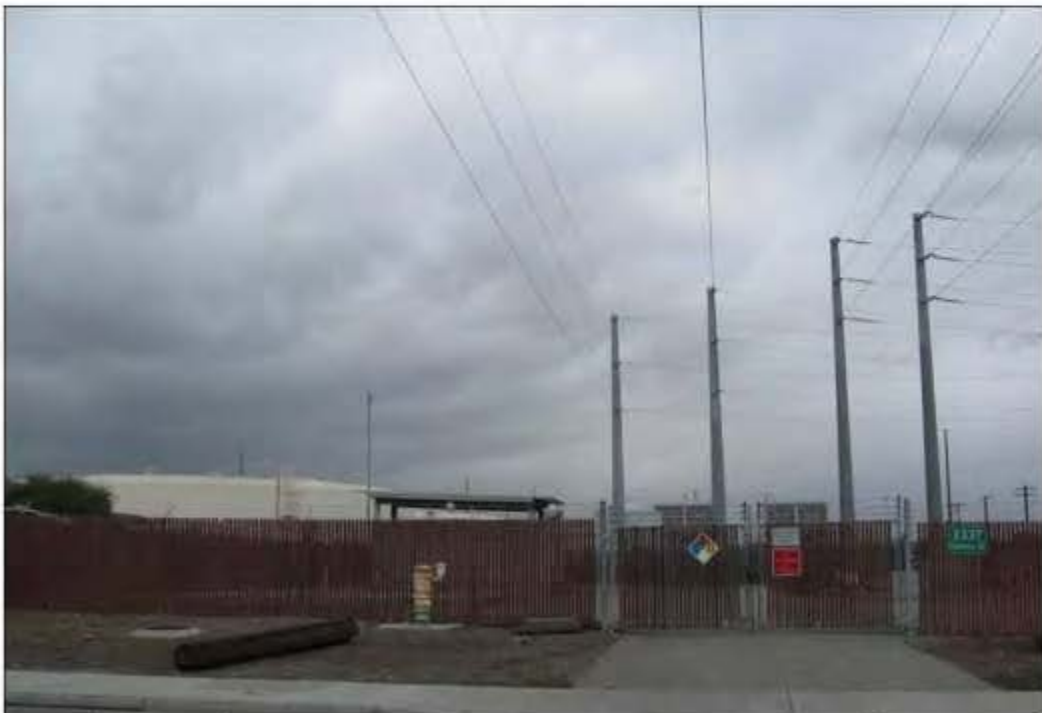
Photo 14 - View of the receiving station and water tanks, looking north from Gianera/6th Street.
