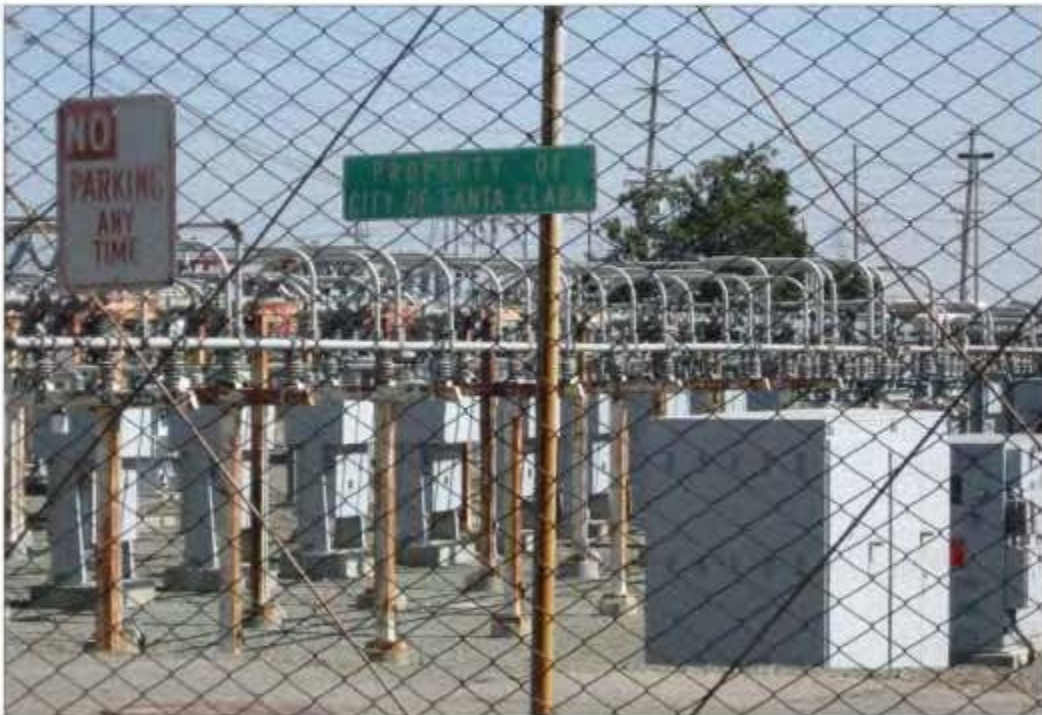
Photo 2 - View of the existing substation, looking south from Tasman Drive.
