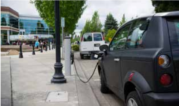
On-street EVCS (parallel space)
