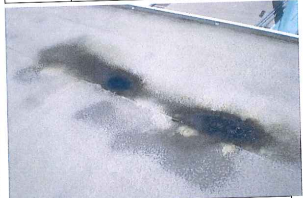
#4: WORN AREAS OF ROOF COATING
