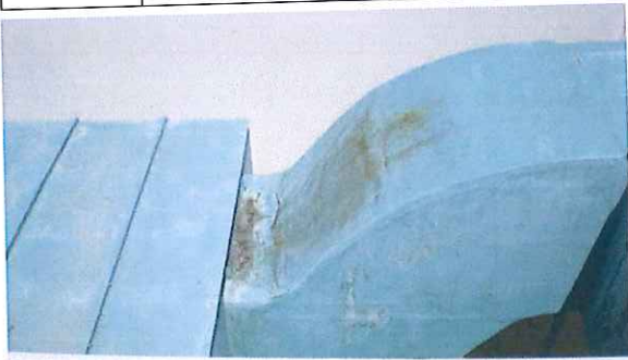
#3: DETERIORATION AT EXPOSED DUCTWORK ON ROOF
