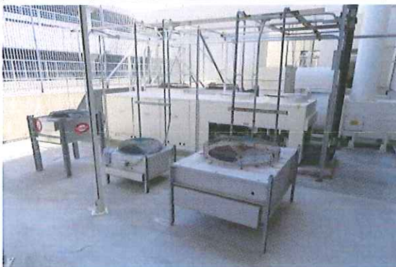
#17: COMMERCIAL KITCHEN, WALK-IN COMBINATION FREEZER/REFRIGERATOR
