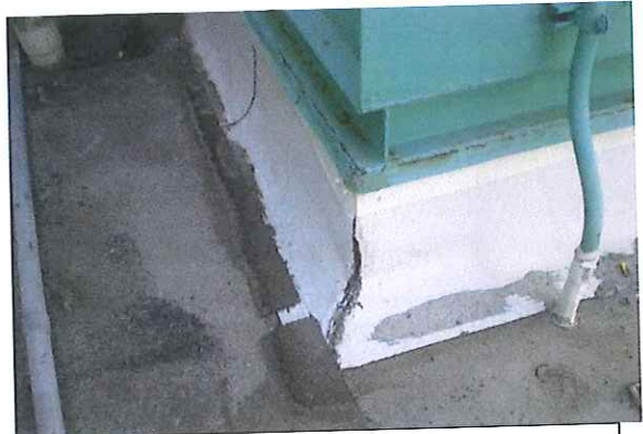
#2: MINOR CRACK AT HVAC EQUIPMENT
