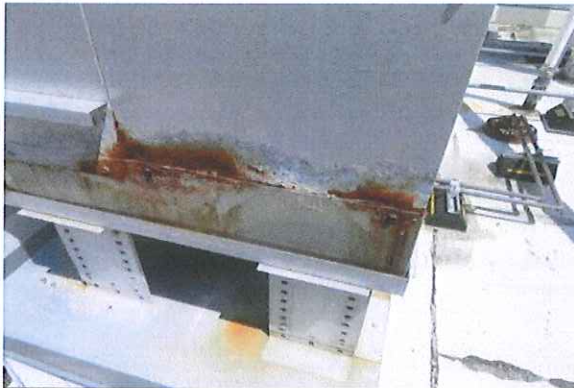
#19: MAKE-UP AIR UNIT, RUST AT FRAME
