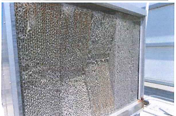
#24: MAKE-UP AIR UNIT, COILS
