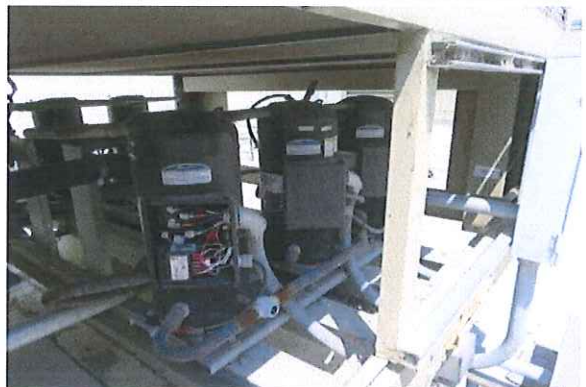
#22: PACKAGED UNIT (RTU)
