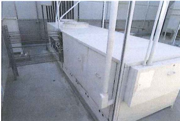
#13: COMMERCIAL KITCHEN CONDENSING UNIT LINKED TO THE ADJACENT UNIT WITH UNINSULATED PIPING
