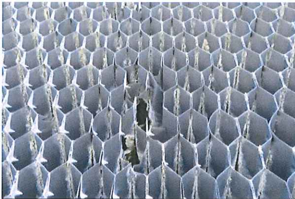
#27: COOLING TOWER CELL DETERIORATION
