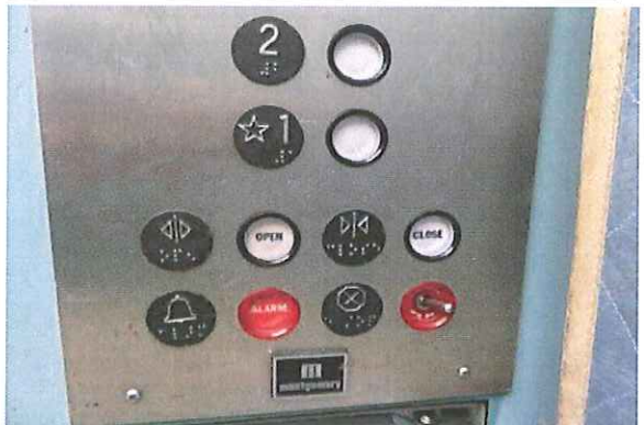
#34: ELEVATOR CONTROLS NOT FULLY COMPLIANT WITH ADA
