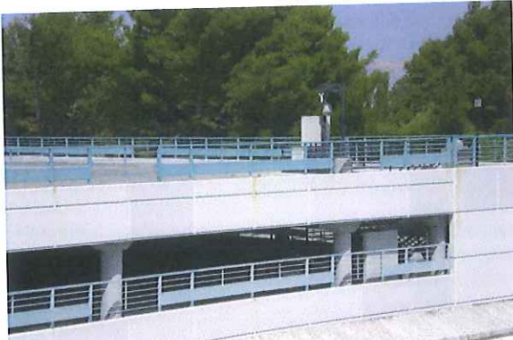
#1: RUST AT PARKING GARAGE WALLS
