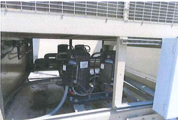
#21: PACKAGED UNIT (RTU)
