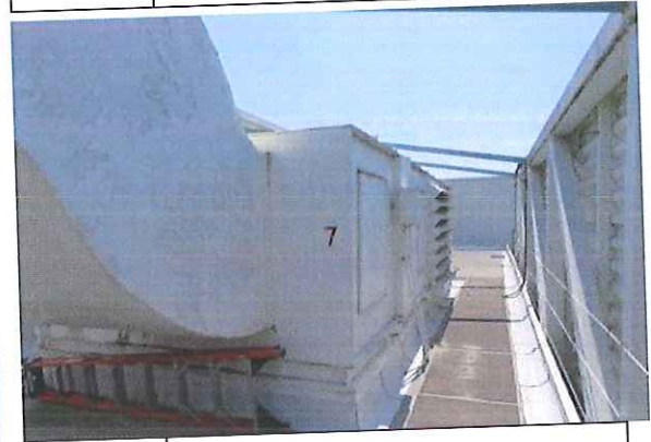
#12: AIR HANDLER, EXTERIOR
