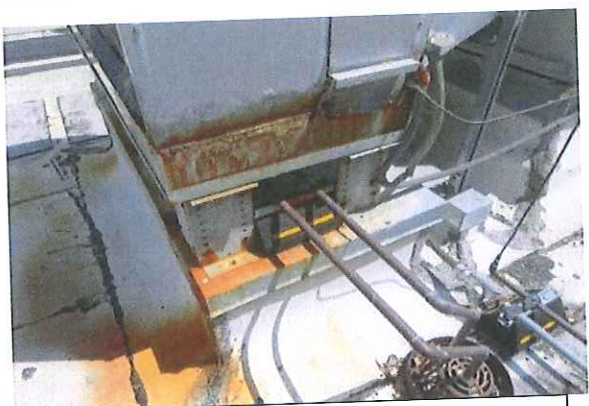
#8: RUST AT MAKE-UP AIR UNIT,
