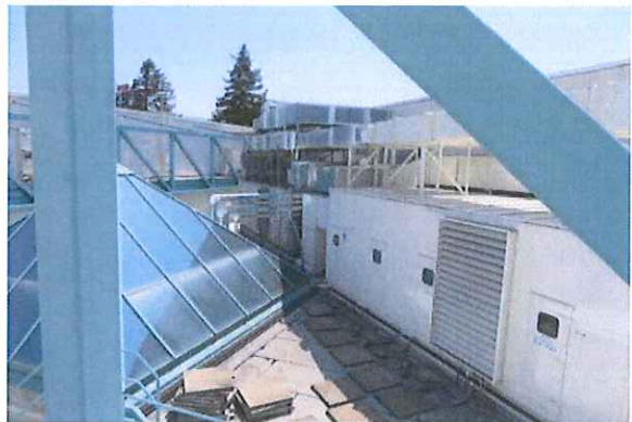
#28: AIR HANDLER INSTALLED TO CLOSE TO SKYLIGHTS
