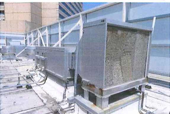
#23: MAKE-UP AIR UNIT COOLING COIL DAMAGE
