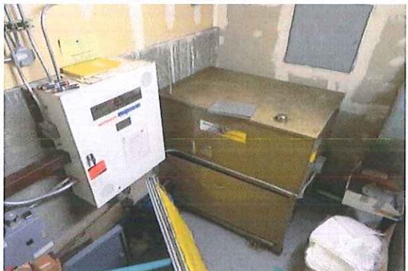
#30: ELEVATOR, HYDRAULIC, EQUIPMENT OBSTRUCTED BY STORED MATERIALS
