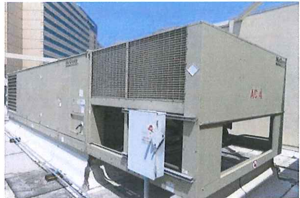
#16: PACKAGED UNIT (RTU)
