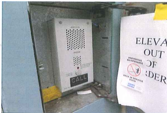
#31: ELEVATOR EMERGENCY VOICE UNITS
