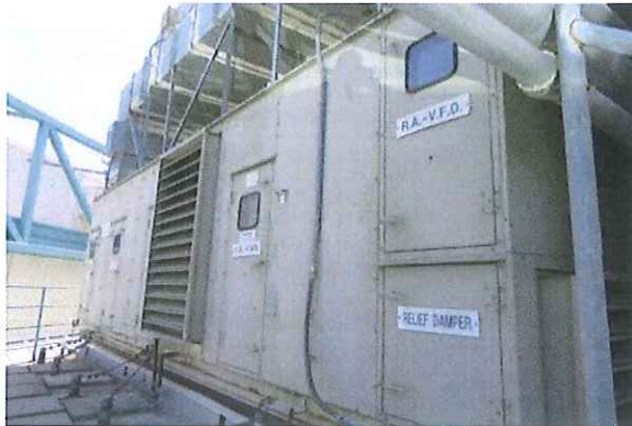
#25: AIR HANDLER, EXTERIOR
