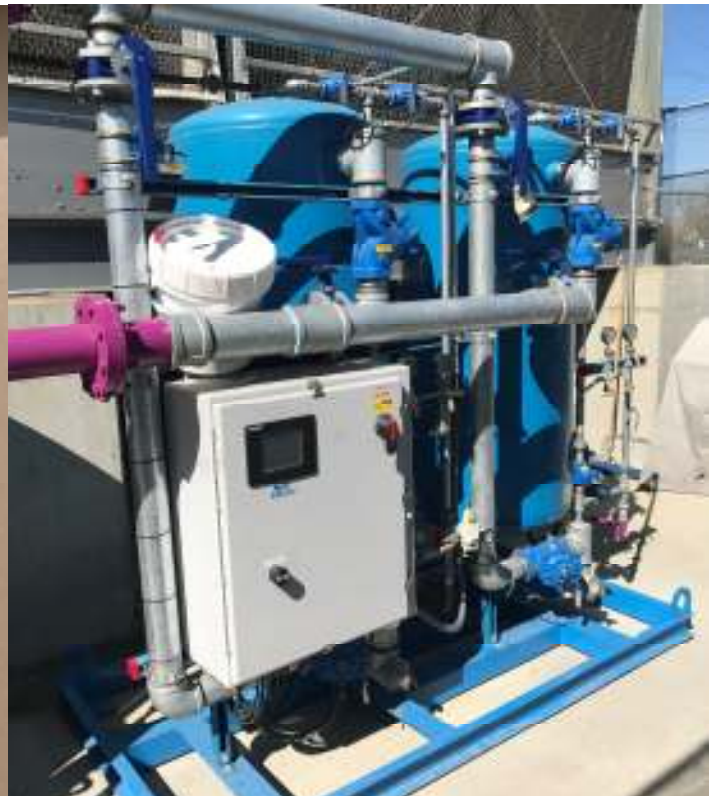
Water Treatment/Softener System
