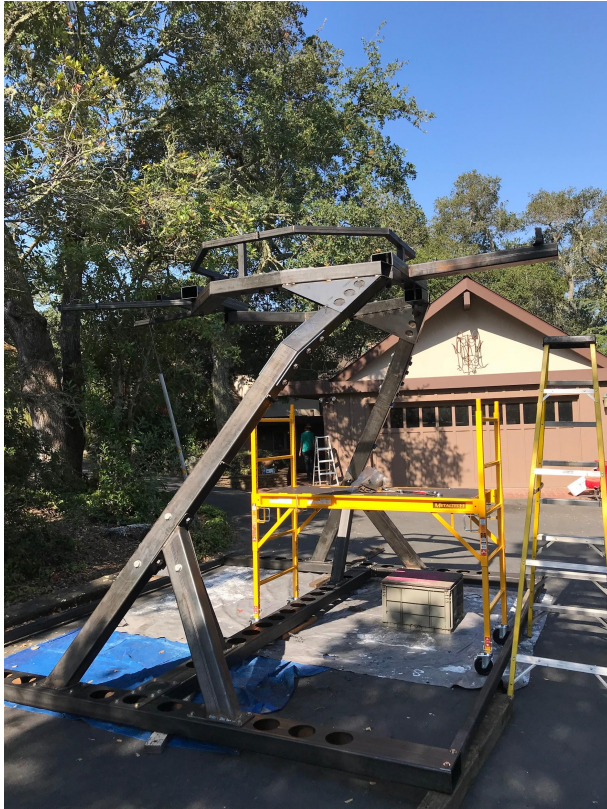
The internal steel frame weighs ~1900lbs, providing a rigid stable base.
