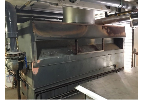
Swim Center Boiler
