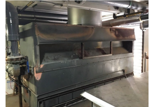
Swim Center Boiler
