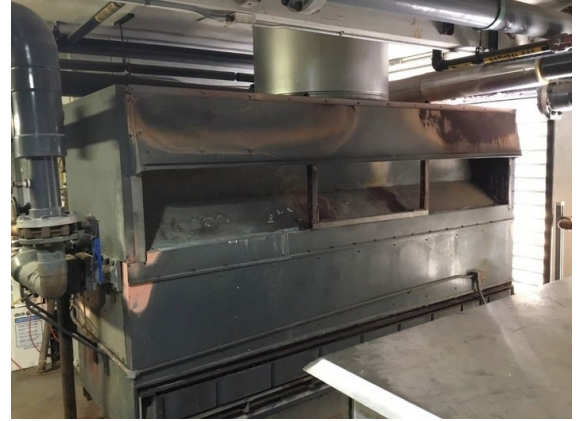
Swim Center Boiler
