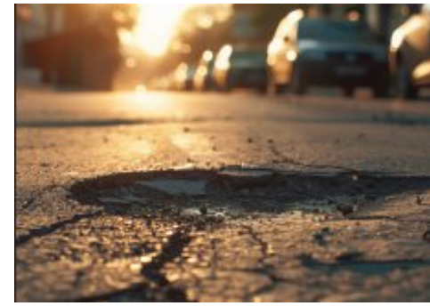
Poor pavement conditions
